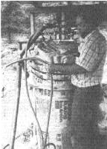
Me draining off trapped air with a hose connected to hose bibs installed at the highest points of the pipes leading to and from the panels.
