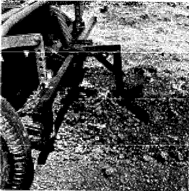
Start moving again and check if the ridge standard is vertical. If it is not, as shown here, ...
