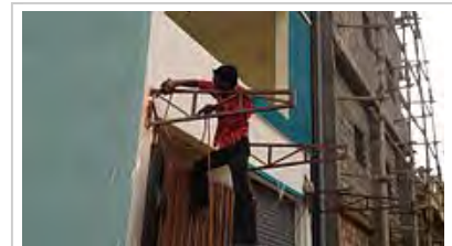
Man welding a metal structure in a newly constructed house in Bengaluru, India
