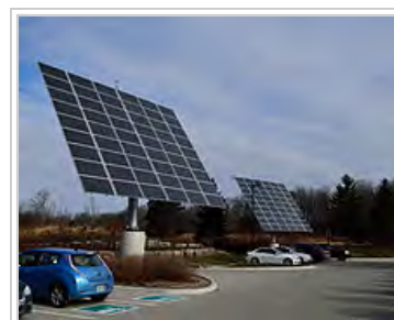
A solar energy charging station in North America
