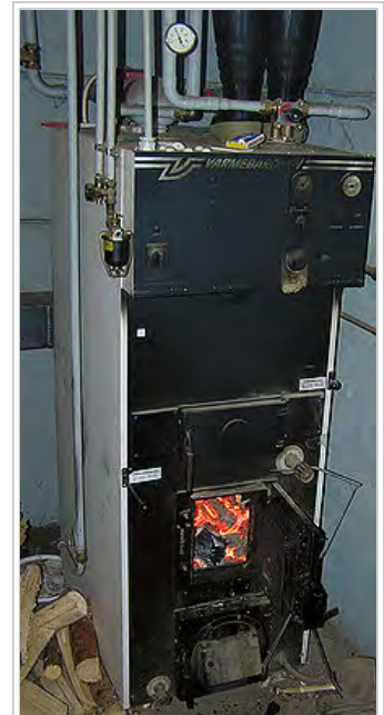
Central heating unit
