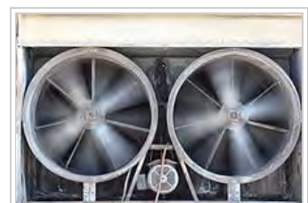
HVAC ventilation exhaust for a 12-story building
