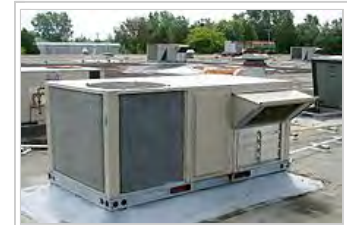
Rooftop HVAC unit with view of fresh air intake vent.
