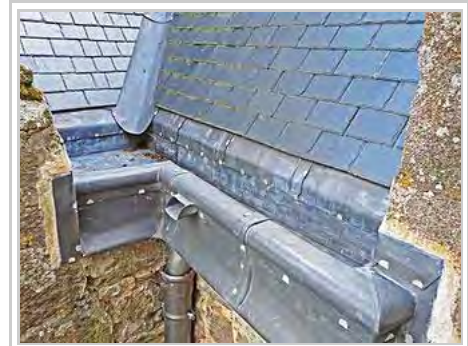
Lead guttering: slate and pitched valley gutter flow into parapet gutter, with downpipe and overflow
