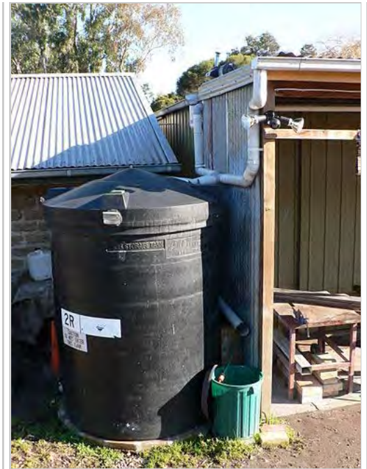
Some of the rainwater tanks around CERES Community Environment Park, in Melbourne, Australia.
