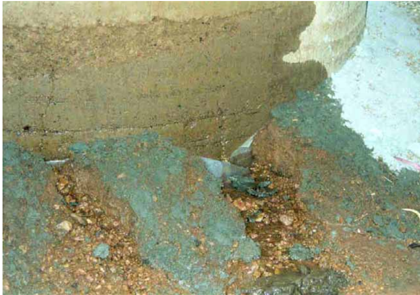
Figure 7.11 Failure of RE2 through 'piping' – this figure shows the leakage at the base of the tank and the crack running through the wall
