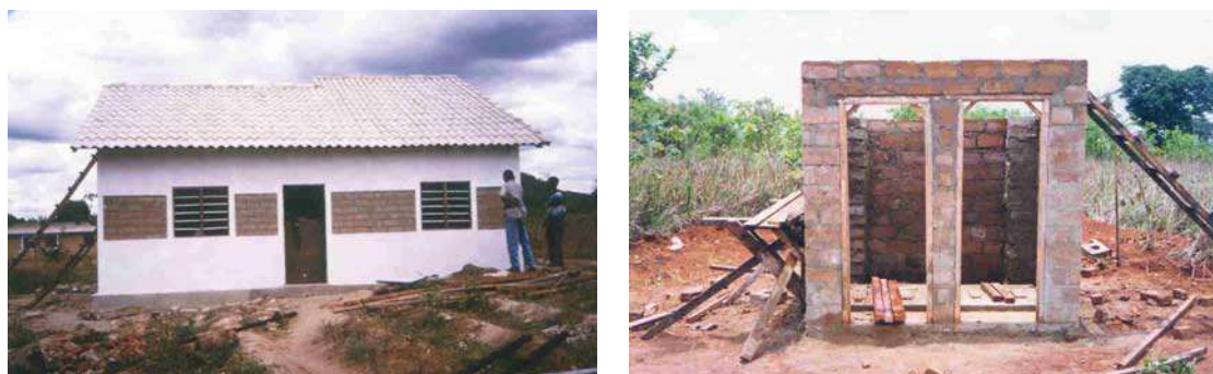
Figure 2.1 Buildings (a clinic and a latrine under construction) made from stabilised soil blocks in Tanzania
