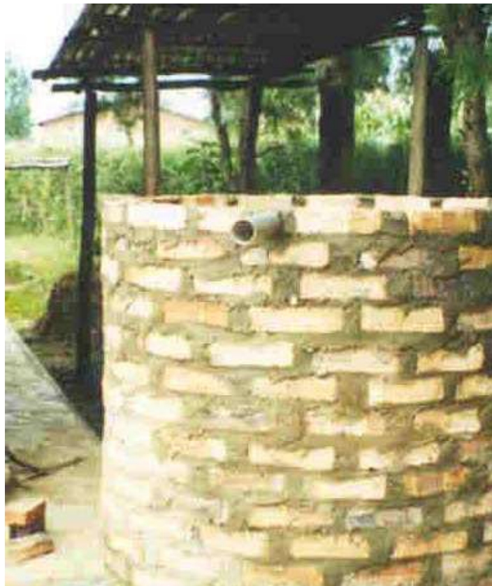
Figure 4 Full height of the brickwork clearly showing the position of the overflow
