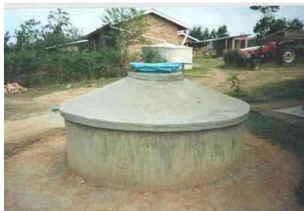
Figure 20 – A completed cover fitted on a partially below ground tank in Uganda
