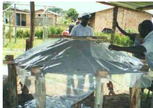
Figure 18 – Curing the cover under plastic. The cover is wetted regularly during curing.
