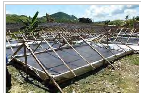
Drying bed for emergency septage treatment by Oxfam in the Philippines
