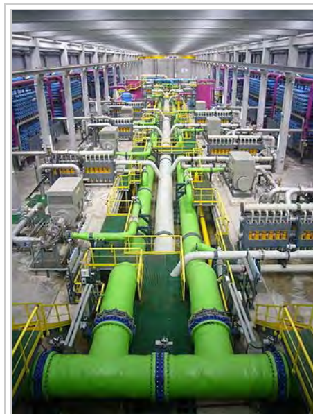
Reverse osmosis (RO) desalination plant in Barcelona, Spain
