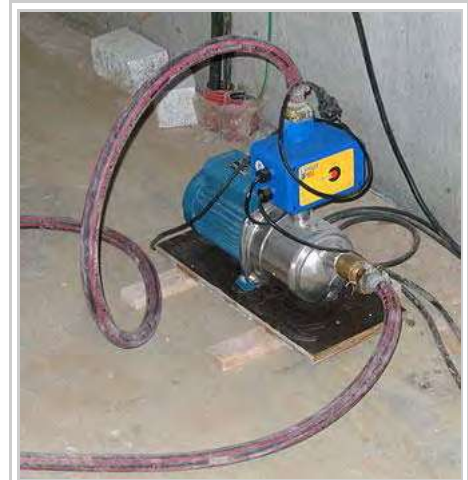
A small, electrically powered pump
