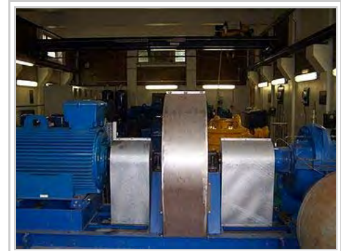
Interior of a water pumping station
