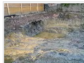
Excavation showing soil contamination at a disused gasworks.
