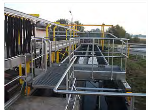
Sand separator in sewage treatment plant in Wieluń.
