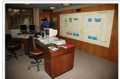
Control room and schematics of the water purification plant to Lac de Bret, Switzerland
