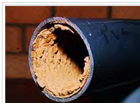
Lime scale in a PVC pipe
