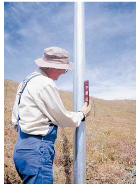
Above: Checking the tower for plumb. The turbine will only yaw properly on a plumb tower.
