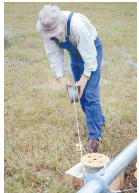
Below: Unreeeling the guy cables. All attachments to the guy bracket are swaged, simplifying assembly.
