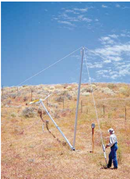
Above: Raising the tower again, this time with the Bergey 850, takes some effort. Going slow allows time for double checking.
