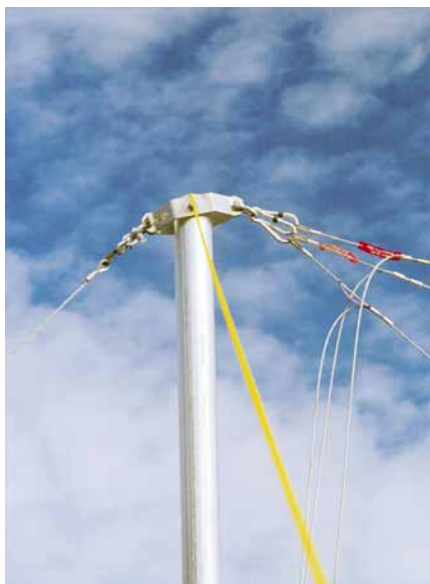
Above: The gin pole bracket showing the hoisting cable (left), nylon rope for steadying, and three lifting guys to tower (right).
