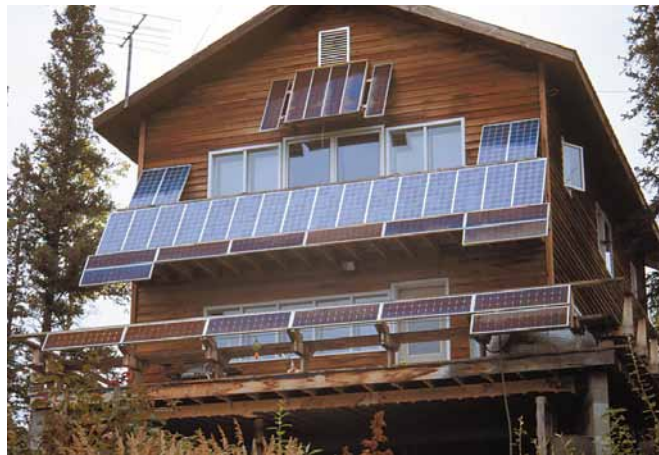
Above: The Dailey home showing off the rest of the RE system.
