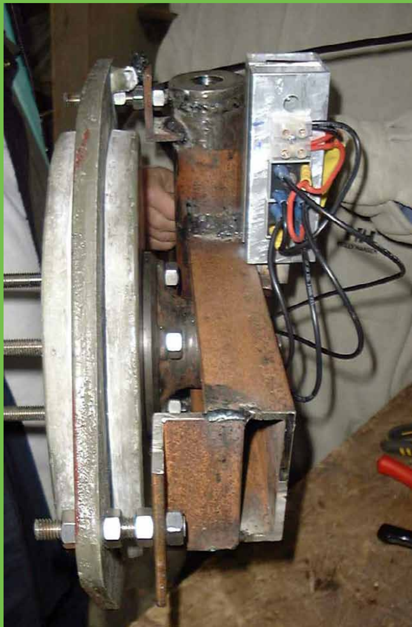
Pic 25: While Julius Tangka is trying to "rip off" the insulation, John and Stephan are checking the tail movement. We had to weld a small additional piece of steel to prevent the tail from hitting the hinge pipe weld.
