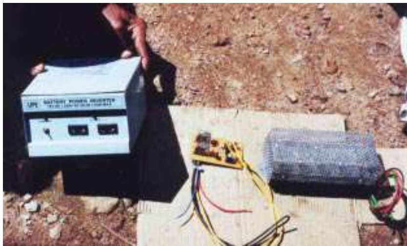
Photo 7: Left to right: Inverter, charge control circuit, and dump load, in Sri Lanka. (Simon Dunnett,)
