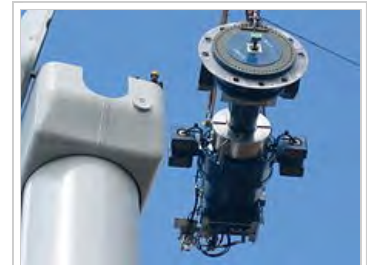
Typical components of a wind turbine (gearbox, rotor shaft and brake assembly) being lifted into position
