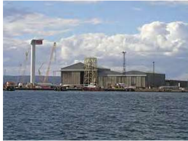
REpower 5 MW wind turbine under construction at Nigg fabrication yard on the Cromarty Firth
