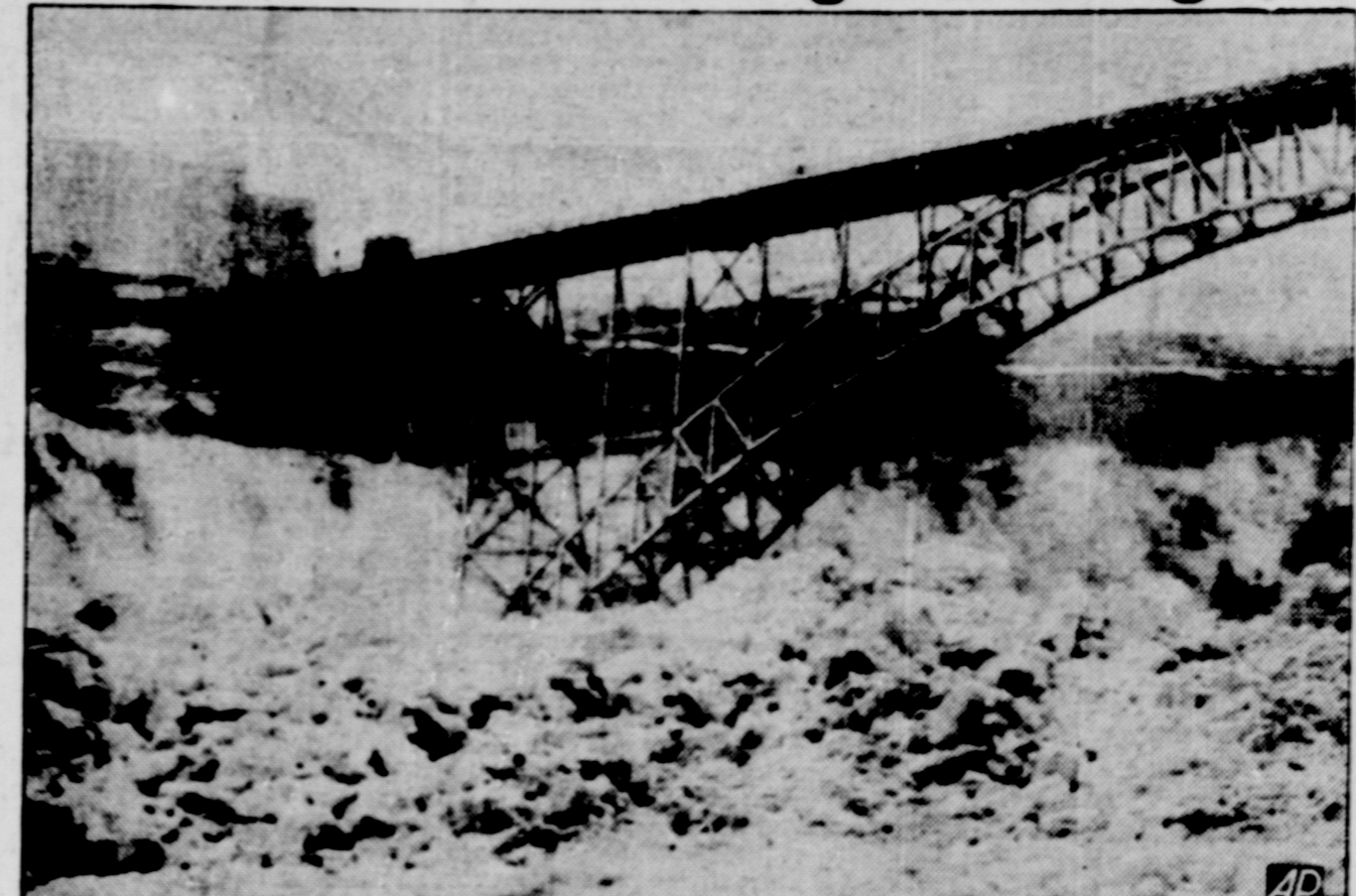
Niagara's famous "Falls View Bridge," high flung steel structure known to millions of honeymooners, wavered dangerously under the onslaught of the biggest ice jam in 30 years. This photo, taken Wednesday, shows the bridge with the pier at the Canadian end surrounded by ice.
