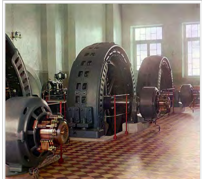
Early 20th-century alternator made by Ganz Works in 1909 in Budapest, Hungary, in the power generating hall of the biggest hydroelectric station of the Russian Empire (photograph by Prokudin-Gorsky, 1911) [1]
