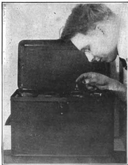
Fig. 20. Examining the Inside of Battery Through the Vent Hole in Top to See the Height of Solution
