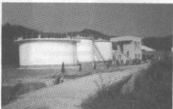
Wastewater treatment plant on a pig farm in Shenzhen City
