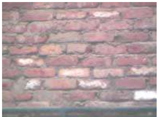
Poorly fired bricks
