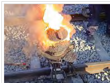
Thermite reaction proceeding for a railway welding. Shortly after this, the liquid iron flows into the mould around the rail gap
