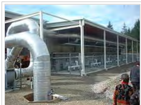
Aeration system for a closed chamber composting facility
