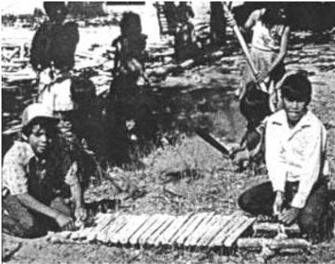
Out of poles they collected from the local forest, school children make a ramp as part of the equipment for the playground.
