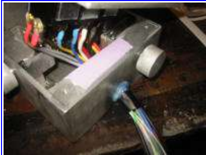
(4) Blue RTV gasket sealer used to seal around the wires before 2 part RTV was poured into place.
