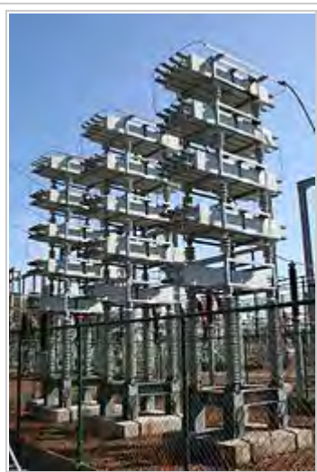
A high-voltage capacitor bank used for power factor correction on a power transmission system
