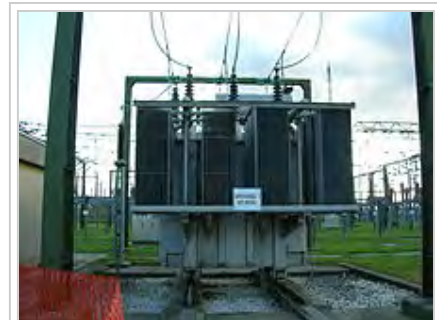
Large 50 MVAR three-phase iron-core loading inductor at an Austrian utility substation
