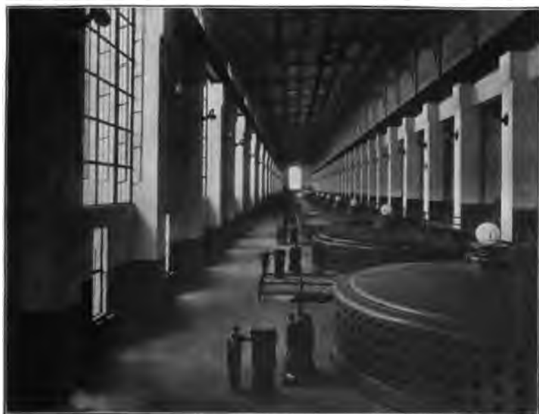
FIG. 291. — Mississippi River Power Company (largest in the world) with fifteen 9000-kv-a. 11,000-volt generators. The ultimate installation will have double its present capacity.
