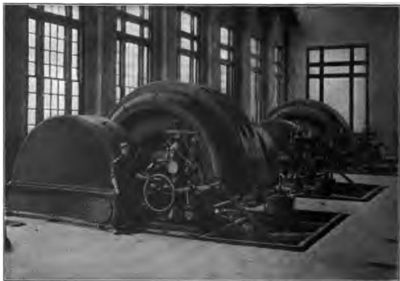
FIG. 292. — Big Creek Development. Power station No. 1. Hydraulic head 1900 feet. Two 17,500-kv-a. 6600-volt generators, each having a momentary peak capacity of 25,000 kv-a. Apparatus controlling Pelton water wheel in foreground.
