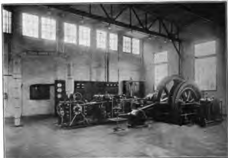
FIG. 289.—Compound Corliss engine connected directly to an a-c. generator. Belt-driven exciter in front, switchboard in rear.
