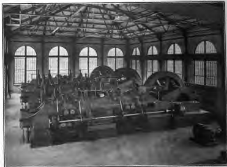
FIG. 290.—Engines using blast-furnace gas. Each engine has two cylinders set end to end, the two pistons being on one long piston rod running through both ends of each cylinder.
