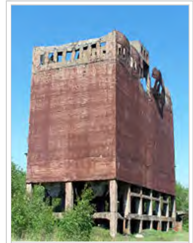
Ruins of the German synthetic petrol plant (Hydrierwerke Pölitz – Aktiengesellschaft) in Police, Poland
