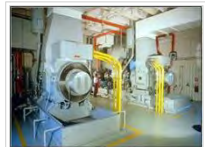
Gas turbines that utilize landfill gas. [8]
