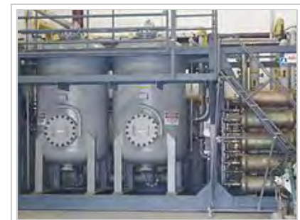
Gas separator membrane skid used in membrane separation process to extract carbon dioxide [13]
