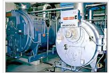
Boiler retrofitted to accept landfill gas. [8]
