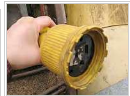
50 amp, 250 volt unloader power socket, with shroud to keep out debris.
