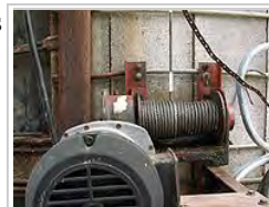
Electric winch for raising and lowering silo unloader.
