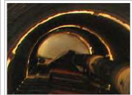
View of the silo unloader drop chute inserted into the very top of the silage drop tube 60ft up. The tube is illuminated by light entering through fiberglass panels every 20ft along the outer steel shroud.
