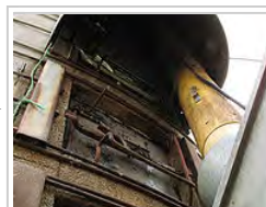
View of silo unloader doors, silage drop tube, and paddle conveyor leading into barn.
