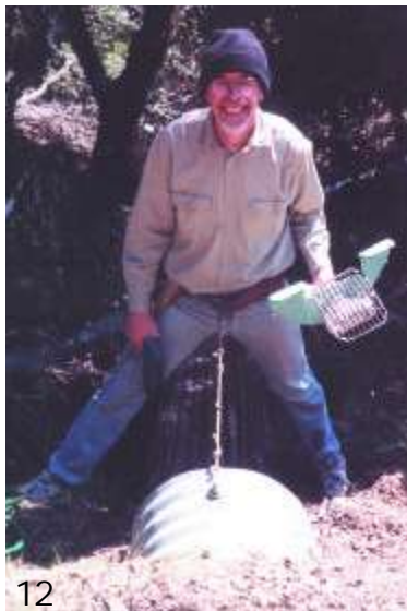
12. With my old tower safety belt secured to a bolt I had added to the northern culvert, I worked hands-free adding the culvert dam.
