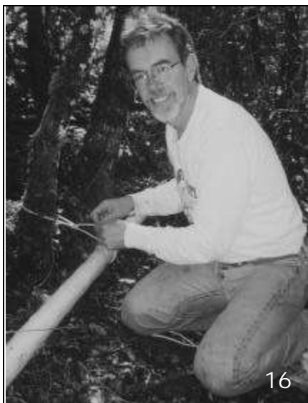
16. The pipe track is secured every 10-15 feet with nylon rope. Don't bind it tight to the anchor point.
