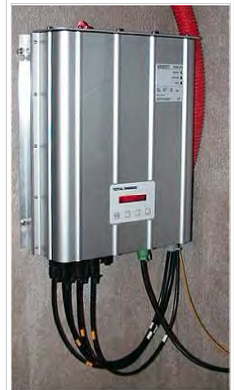
Inverter for grid-tied solar panel
