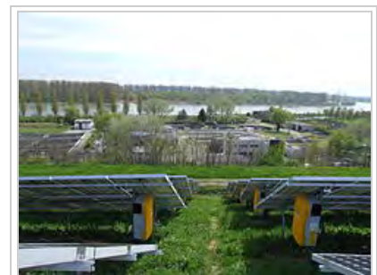
Overview of solar-plant inverters
