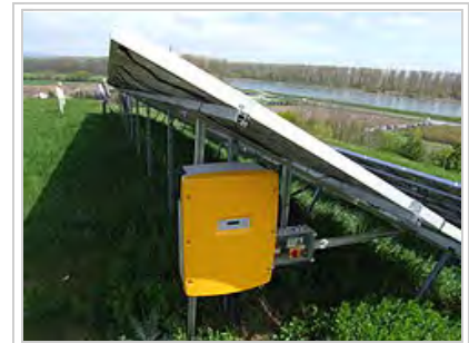
An inverter on a free-standing solar plant
