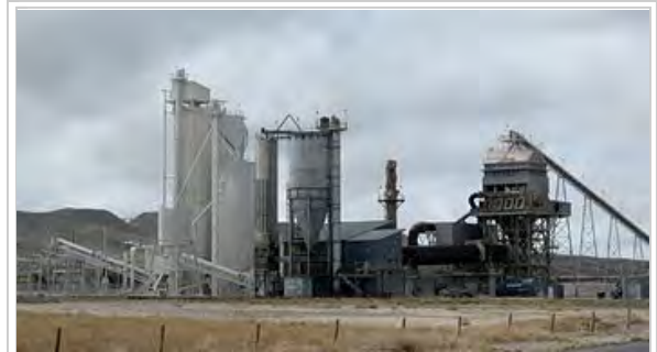
Rotary lime kiln (rust-colored horizontal tube at right) with preheater, Wyoming, 2010
