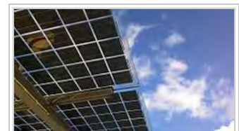
Double glass photovoltaic solar modules, installed in a support structure.
