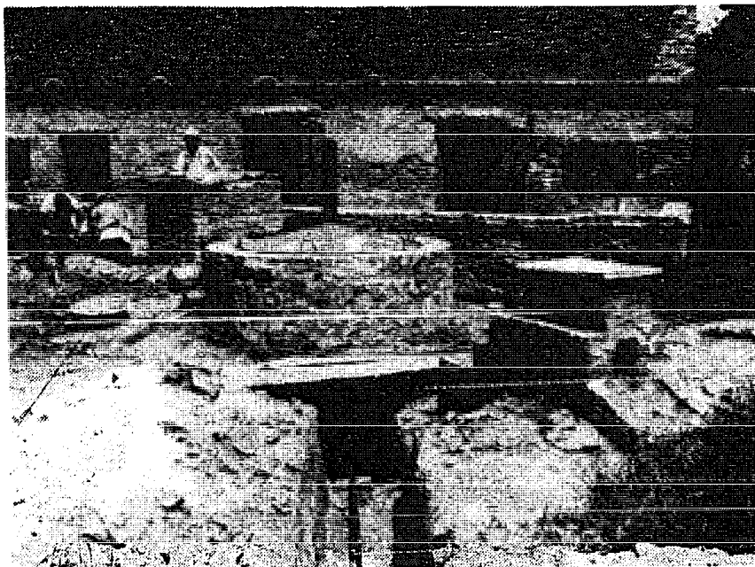
One of the first private gas plants in Kathmandu nearing completion. It is five metres deep and 180 cm in diameter. Notice the mixing trough behind pit, outlet (right foreground) and gas pipe to kitchen.
