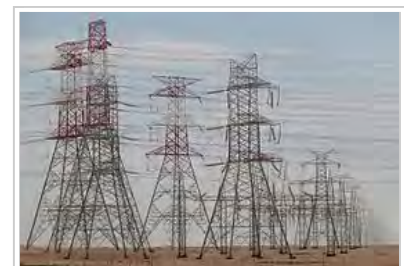
Power lines in Qatar
