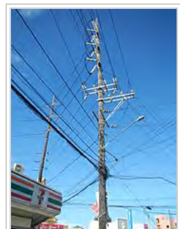
A 115 kV subtransmission line in the Philippines, along with 20 kV distribution lines and a street light, all mounted in a wood subtransmission pole
