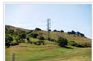
A high-power electrical transmission tower, 230 kV, double-circuit, also double-bundled
