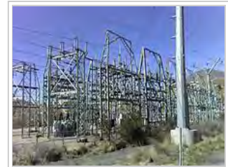
A transmission substation decreases the voltage of incoming electricity, allowing it to connect from long distance high voltage transmission, to local lower voltage distribution. It also reroutes power to other transmission lines that serve local markets. This is the PacifiCorp Hale Substation, Orem, Utah, USA
