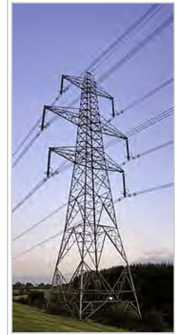
Two-circuit, single-voltage power transmission line; "Bundled" 4-ways
