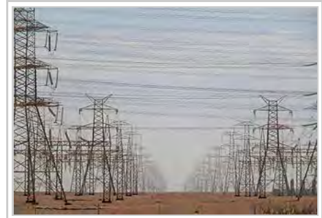
Transmission lines transmit power across the grid.
