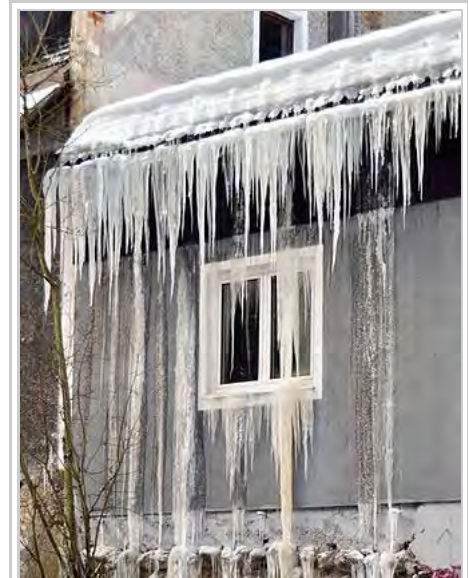
Icings resulting from water leaking through the roof due to an ice dam, caused by snowmelt on the roof.
