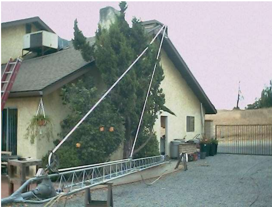
You can see how this works. There is a double pulley (2 grooves side by side) on the roof.
