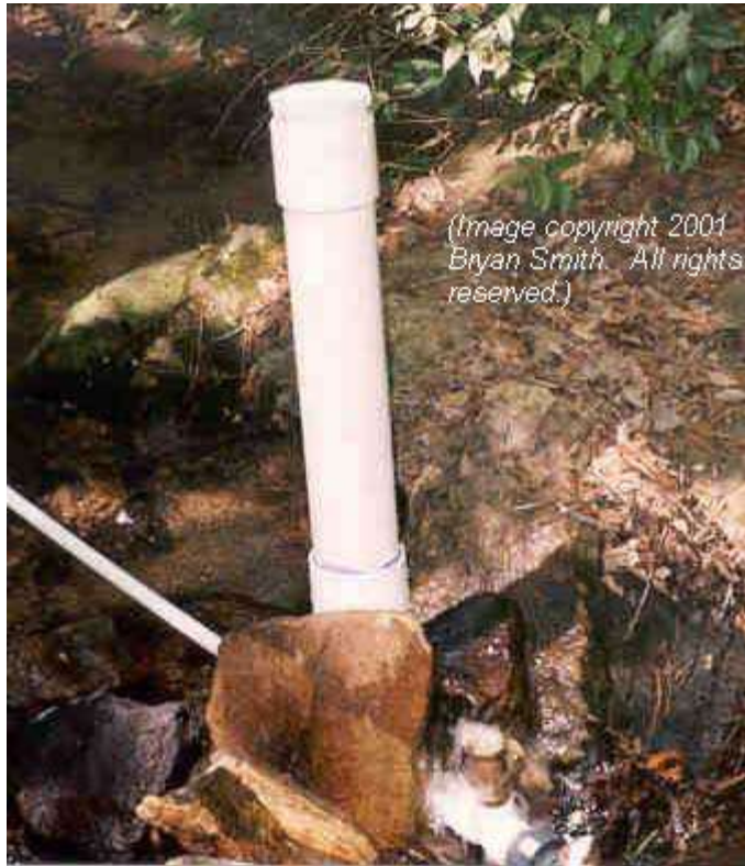
Figure 1. The ram pump installed and operating. Note the water exiting the waste valve and the rock used to hold the pump upright and anchor it.
