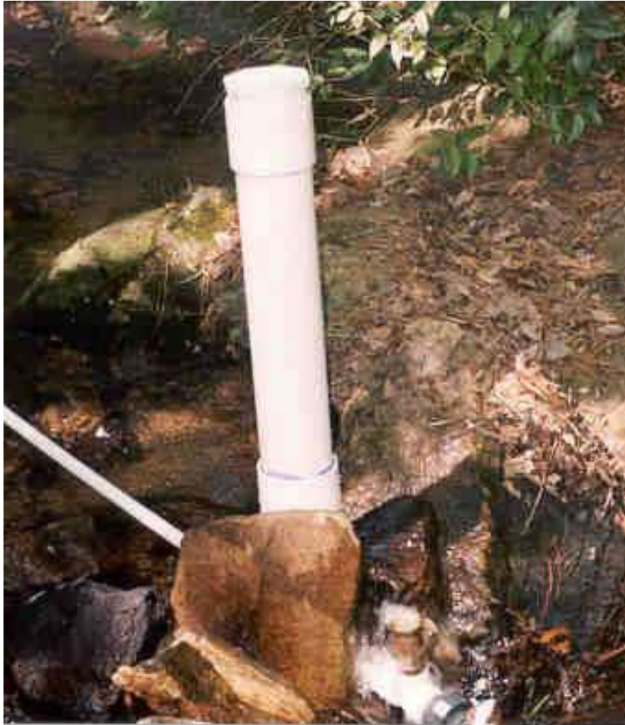
Figure 1. The ram pump installed and operating. Note the water exiting the waste valve and the rock used to hold the pump upright and anchor it.
