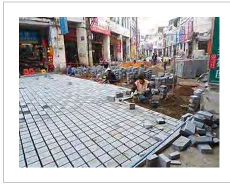
Replacing the old road with concrete blocks in Bo'ao Road area, Haikou City, Hainan, China
