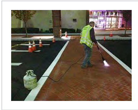
Polymer cement overlaying to change asphalt pavement to brick texture and color to create decorative crosswalk
